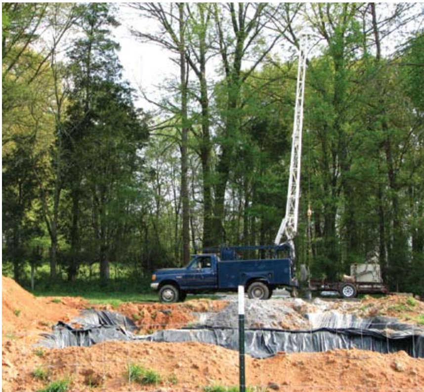
Core samples being taken from "Coles Hill" in Pittsylvania County near Chatham
